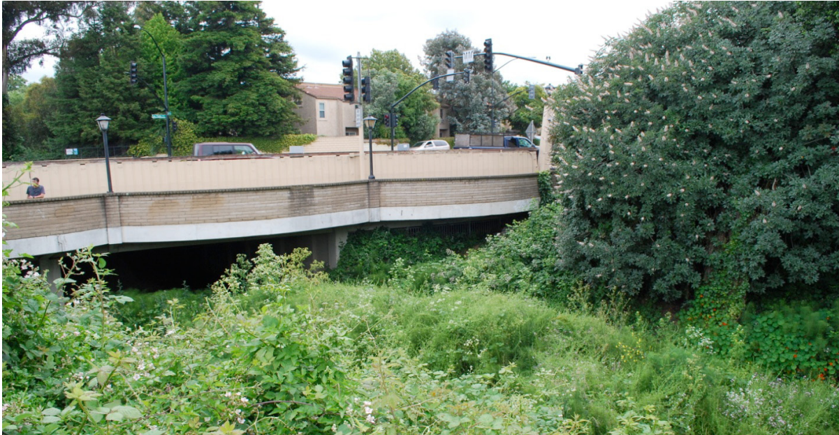
Photo 12: View of the San Pablo Avenue bridge and pedestrian walkway over San Pablo Creek from Road 20 on the north side of the creek.
