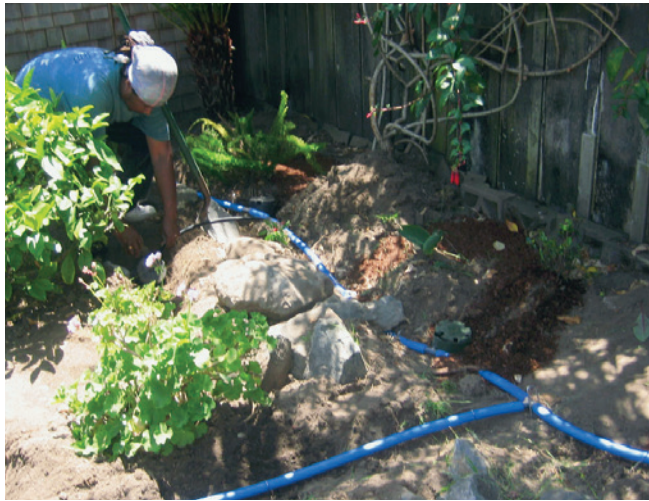
1-inch Blu-lock HDPE tubing laid out in trenches. All tubing is buried after system is installed. Photo: Laura Allen.
