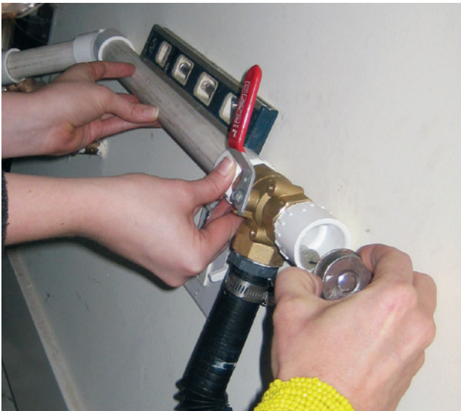
Gluing pipes on either side of a 3-way valve. Photo: Laura Allen.
