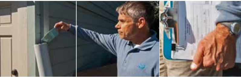
To keep the San Francisco Bay clean, EBMUD inspector Michael Walton conducts private sewer lateral tests to ensure leak-free pipes.
