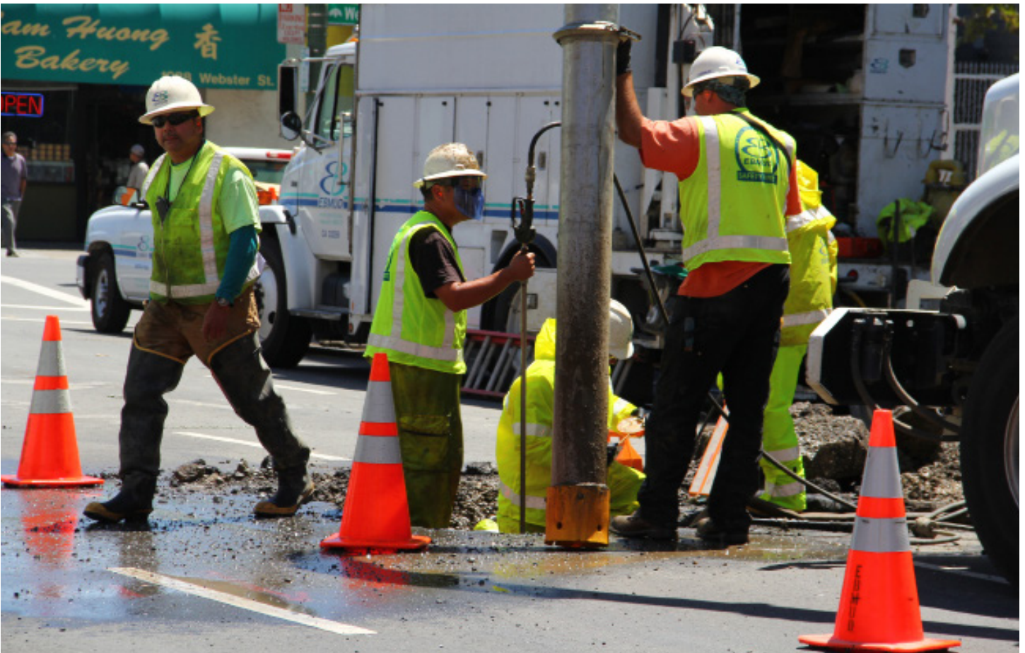
EBMUD crew working on repairing a water main break in downtown Oakland.
