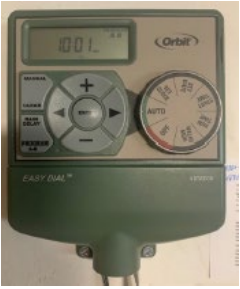
1) Old conventional controller
